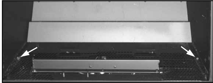
Figure 10: Screws Holding Burner Tray in Place.
